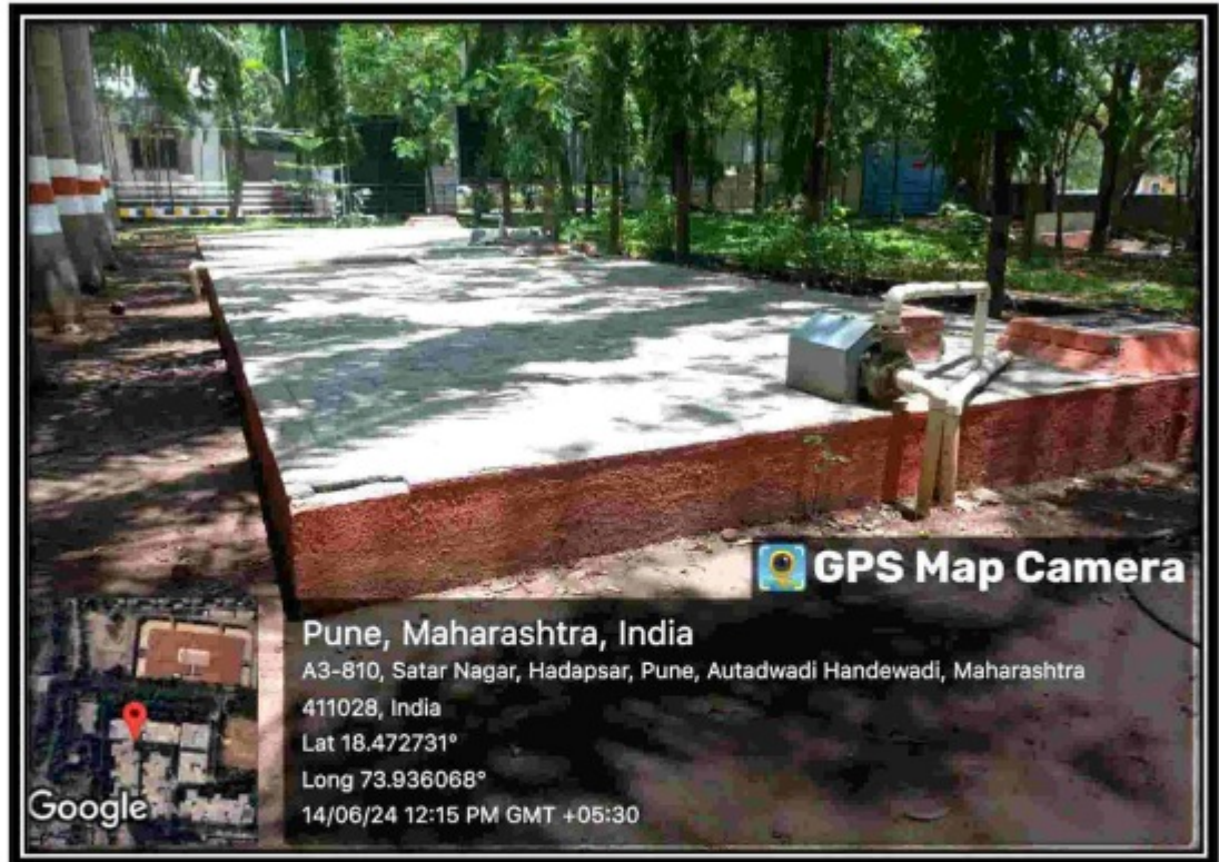
Underground Water Tank
